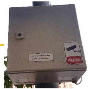
Box with the battery
